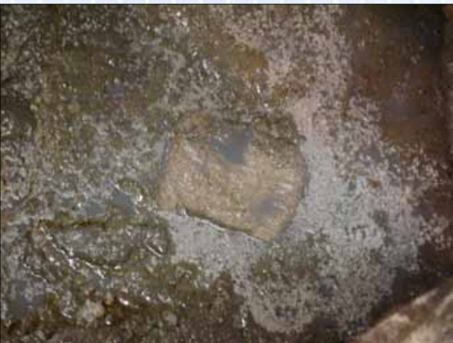
BCP10 water soluble bag breaking down in wastewater system.
